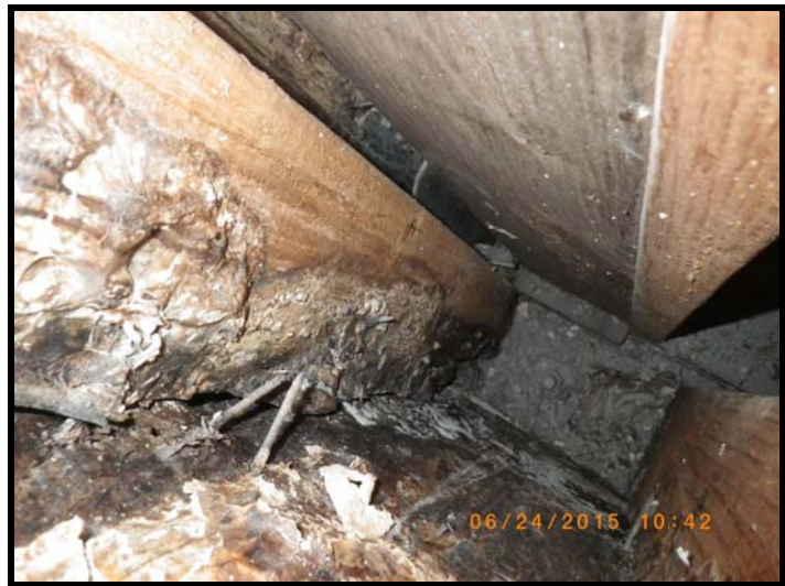
Photo taken after removing the perfectly fine stucco finish of a 3 year old structure in May 2015. This is the support frame for the floor above.
